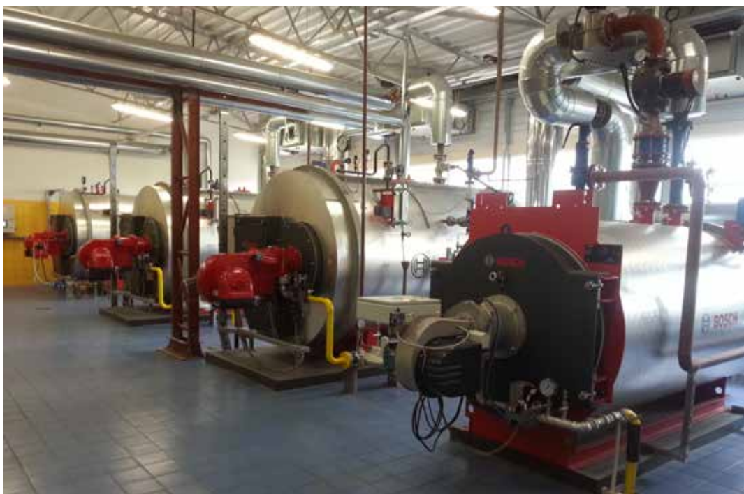
Modernised energy system in Provincial Hospital in Kalisz. Photo Wojciech Grzelak
