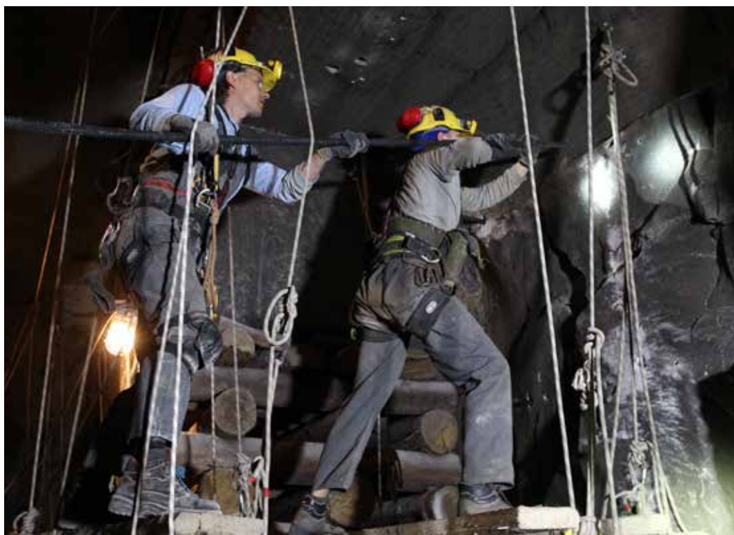
Significant financial contribution of the National Fund was transferred to so abandoned workings in salt and coal mining. Photo Salt Mine „Wieliczka” P. P.
