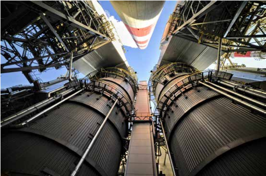
Installation for wet desulphurization and catalytic denitrating of flue gases in CHP Siekierki. Photo Tomasz Banasik
