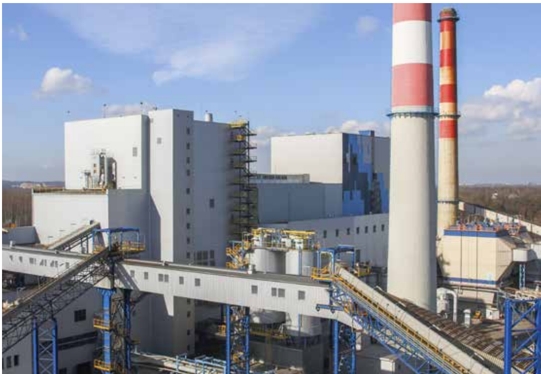
Biomass fired boiler in Jaworzno III Power Plant. Photo Wojciech Piechocki
