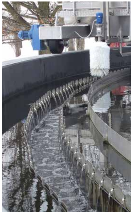
Modernization of sewage treatment plant in Grodzisk Mazowiecki co-financed by EU.
