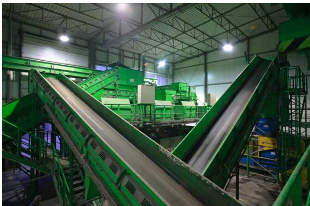
Automatic waste sorting line in Eco-Valley Photo Piotr Wittman
