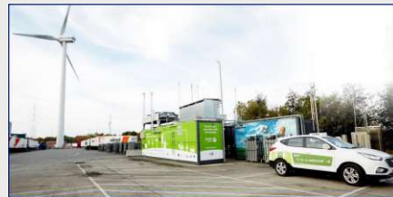
Colruyt Group, Halle (Electrolysis +RE)
