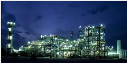
Air Liquide, Port Jerome (SMR +CCS)
