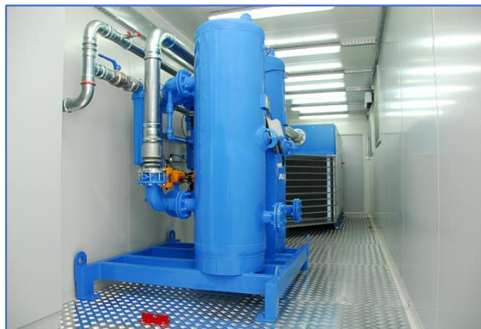
Pic. 1 almig: compressed air installation
