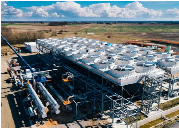
Velika Ciglana, Croatia Geothermal Power Plant
