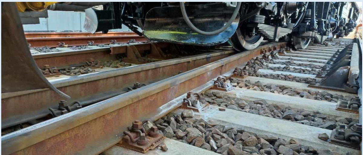
Photograph 26 – Consequences of the occurrence – derailment of locomotive EU07-1529 (source: own material of PKBWK)
