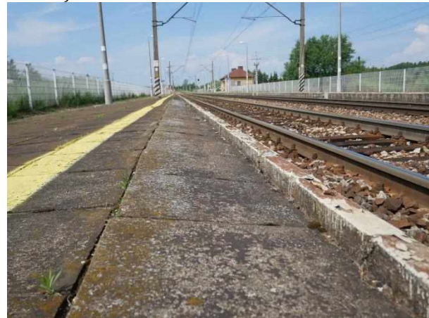
Photograph 3 – A view of Platform 2 with uneven pavement (own material of PKBWK)
