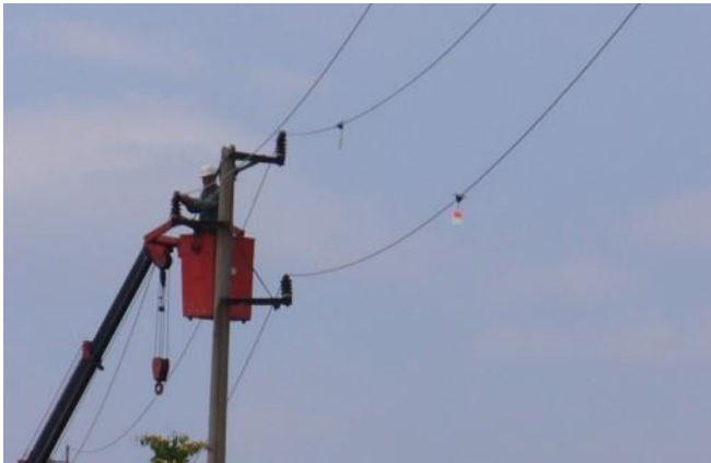
Over 2 000 electrical diverters will be mounted
