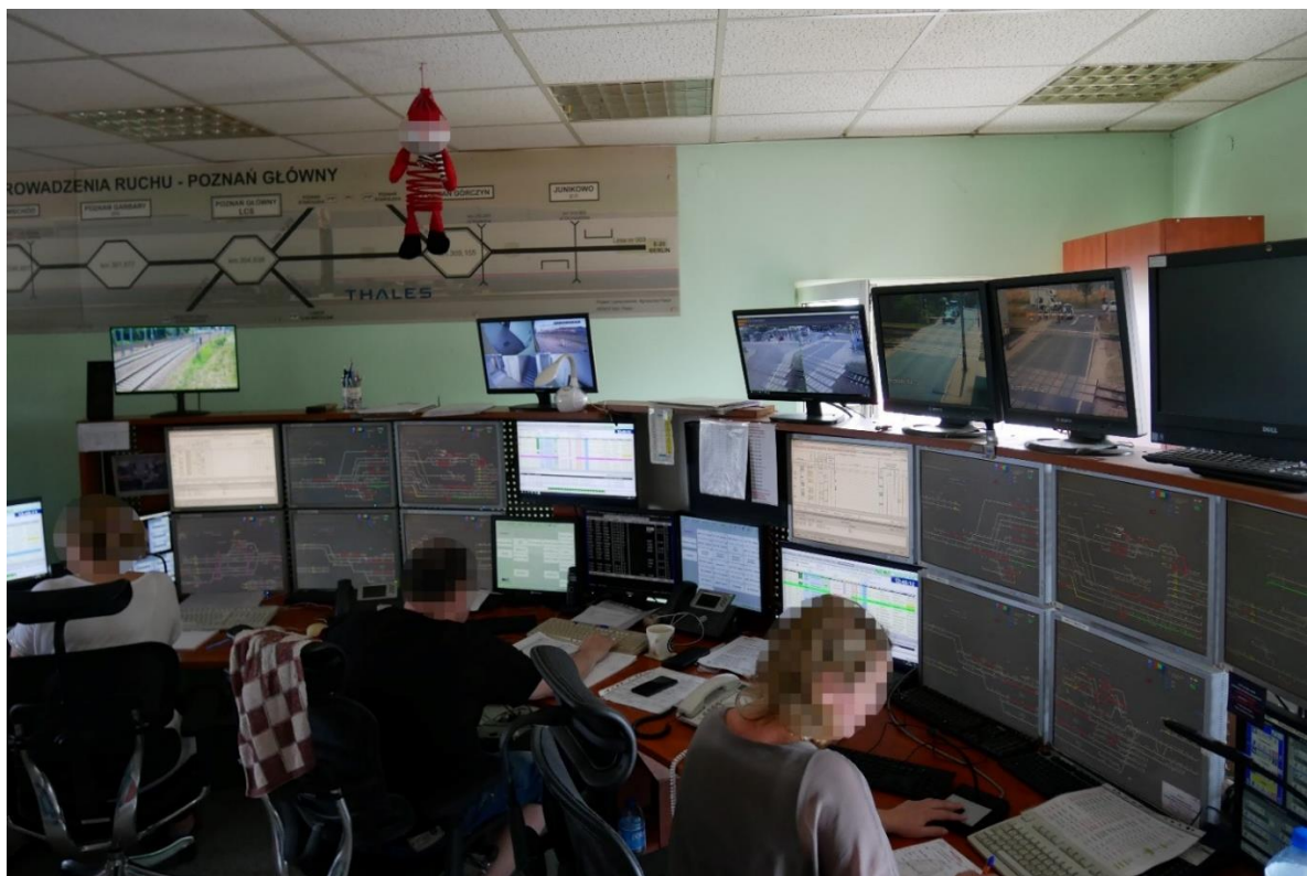
Photograph 6 - Operator stations of signallers C and D, and operating station of the dispatcher
