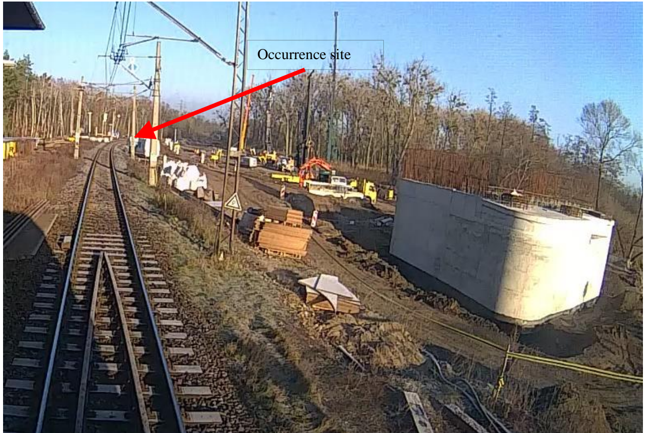
Photograph 3. A general view of the route and the site of the occurrence as seen from the driver cabin in daylight on 19 January 2023. Visible is the construction site whose illumination at nighttime hindered observation of the route by the driver of the rail vehicle (materials of the railway commission).
