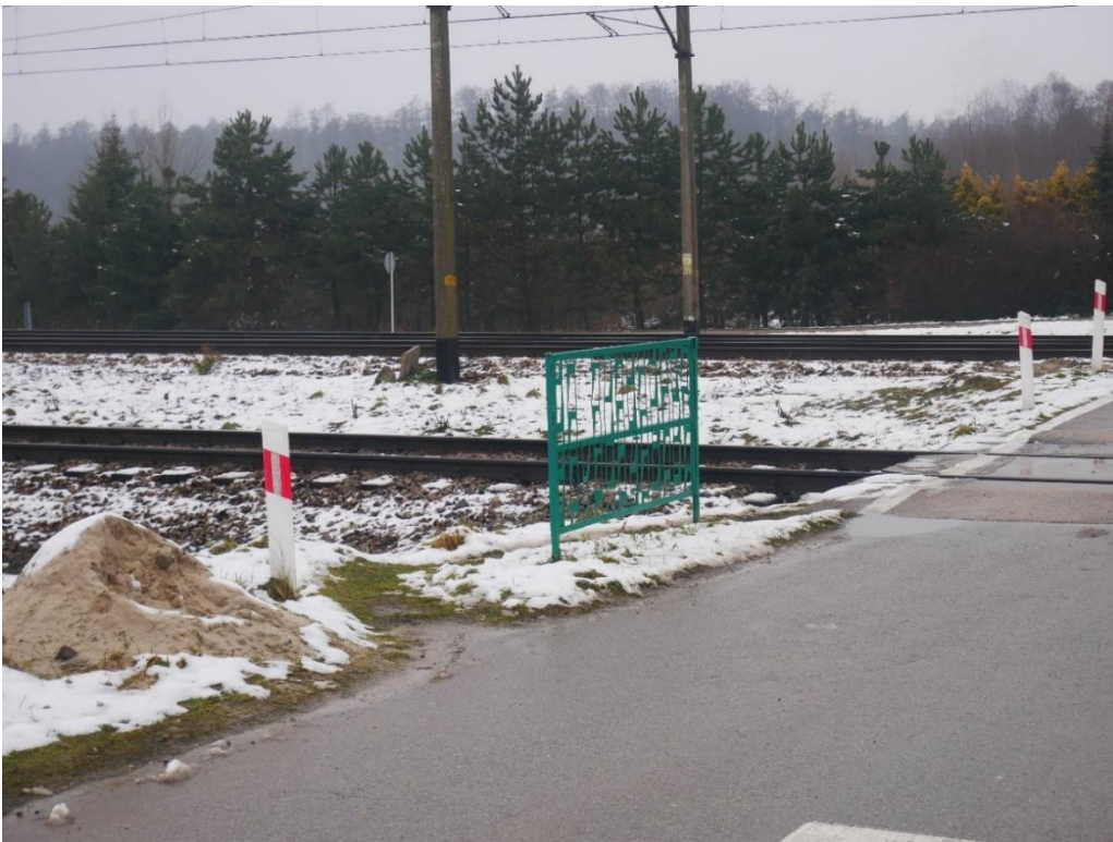
Photo 10 - View of the Cat A crossing km 244.630 with fencing (PKBWK's own material).
