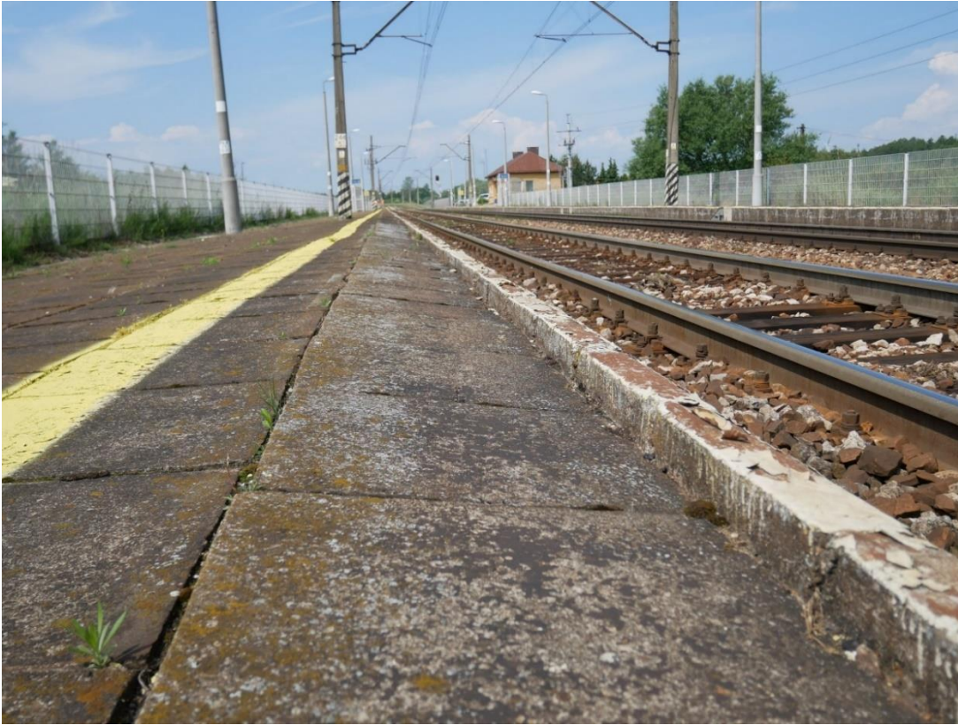
Photo 11 - View of Platform 2 with uneven pavement (PKBWK's own material).
