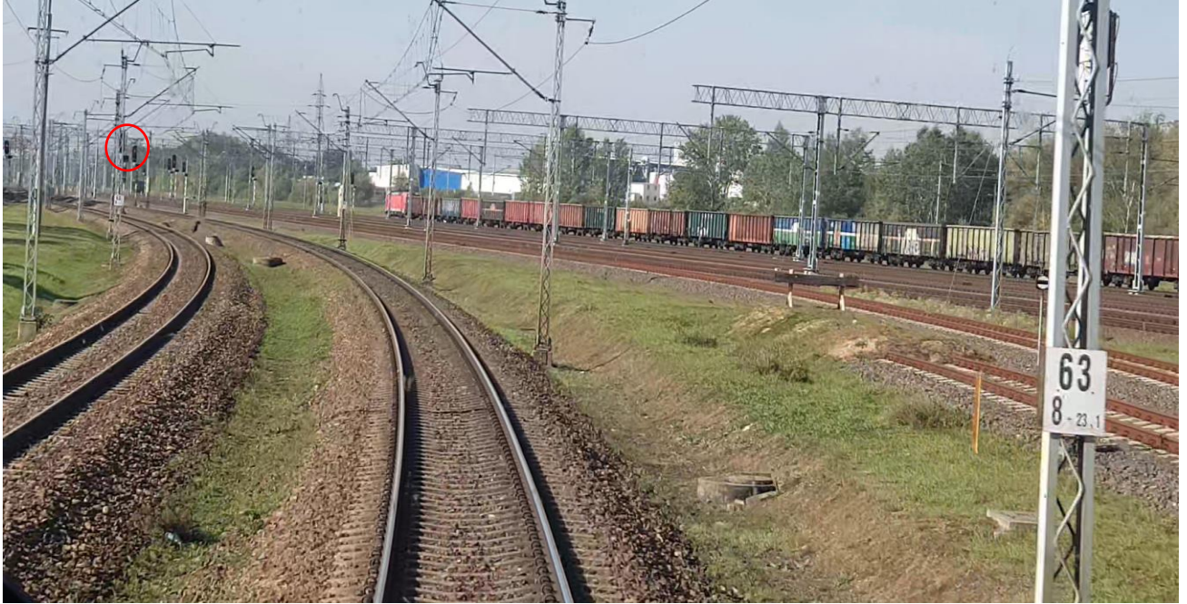
Photograph 11 - A view of the signal J1 1/2/3/m 340 m (own material of PKBWK)
