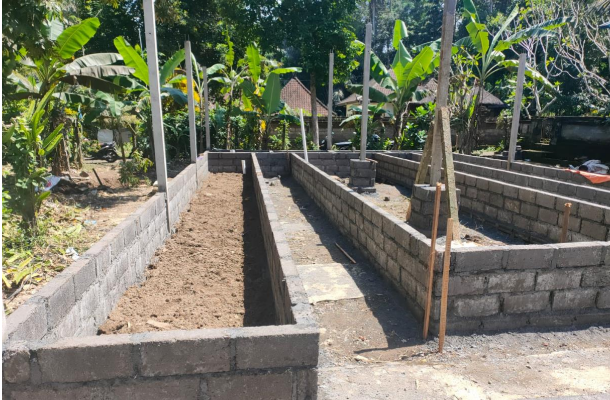
The initial construction process of aquaponic facility by creating a structure of fish pond and water reservoir filtration system
