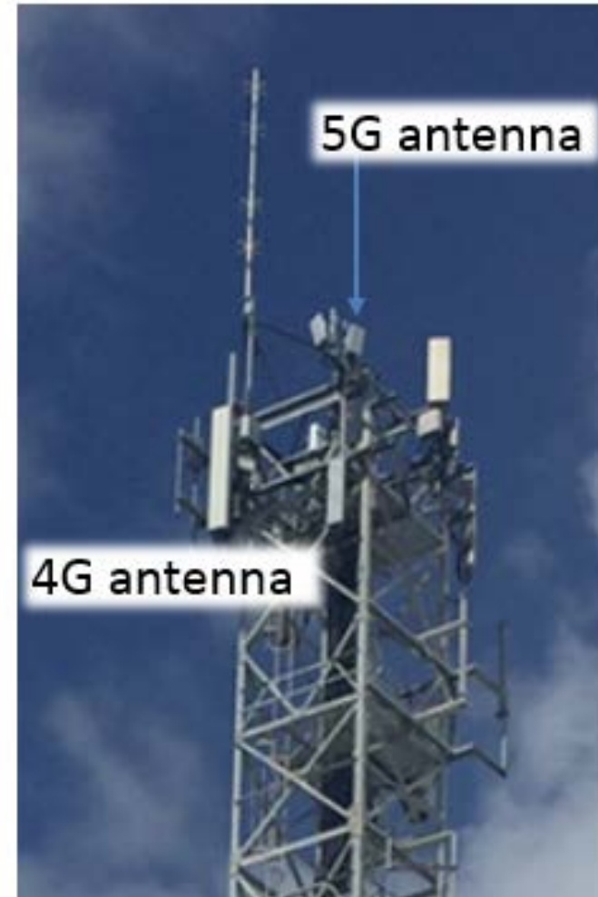
Southport Radio Tower 27GHz mmWave 5G antenna
