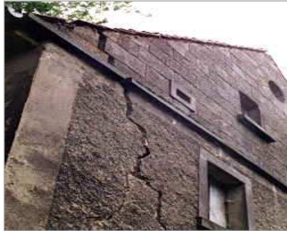
Post-mining ground deformations
