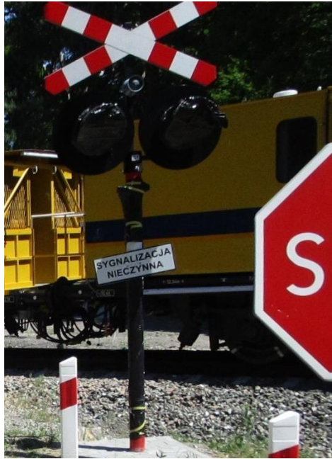
Photograph 7 – “signalling out of order” sign placed on the traffic signal
