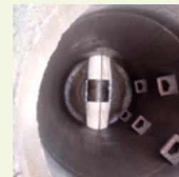
Fig. 16. Renovation of storm water channels by means of on-site hardened sleeve in Bydgoszcz, photo by Jakub Wysocki
