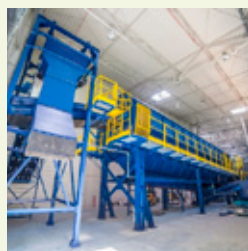
Fig. 28. Fragment of technological line, rotary sieve, photo by FBSerwis Kamieński Sp. z o.o.
