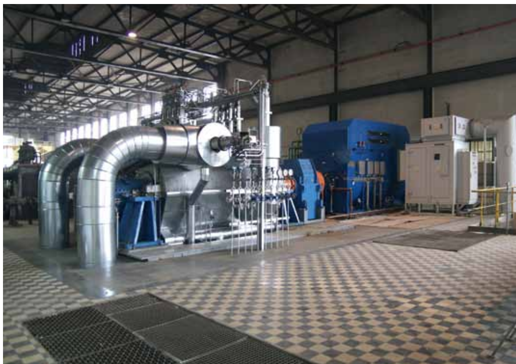
Turbogenerators. Fot. Synthos Dwory 7
