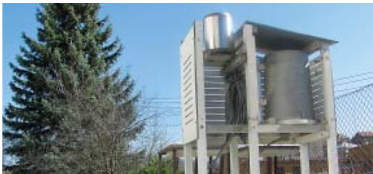
Photo 10. Early warning station for radioactive contamination PMS
