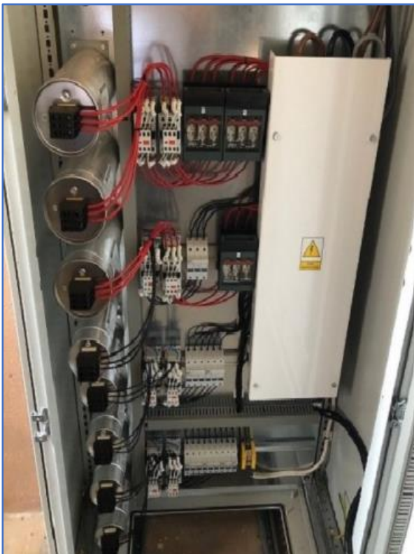
Pic. 1 BMS: capacitor battery for compensating inductive reactive power
