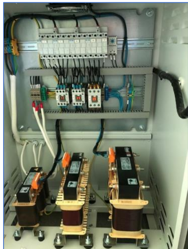
Pic. 2 BMS: choke battery for compensating storage reactive power
