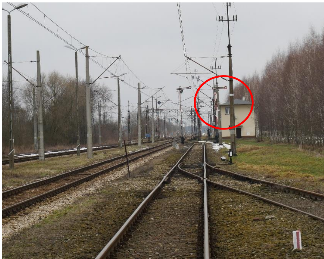
Photo 5 – view of pole hiding the night signal of semaphore D (photo by PKBWK)
