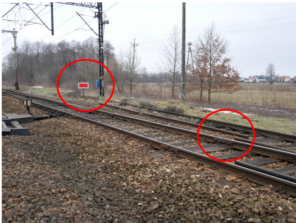
Photo 6 – closed track 3 and discontinuity of track 3 beyond the crossroad of turnout no. 3
