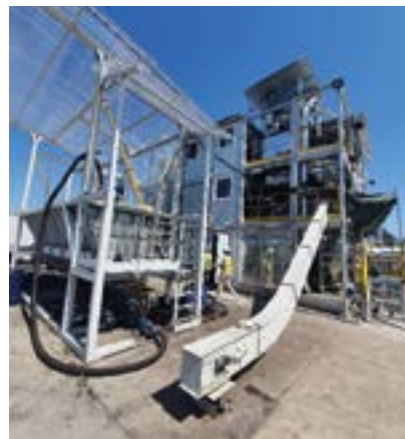
■ ZEWERO plant (gasification of sewage sludge)
