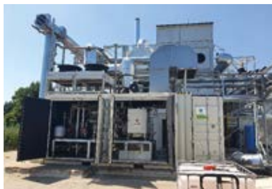
■ ZEWERO installation (gasification of sewage sludge) – gas-fueled power generator
