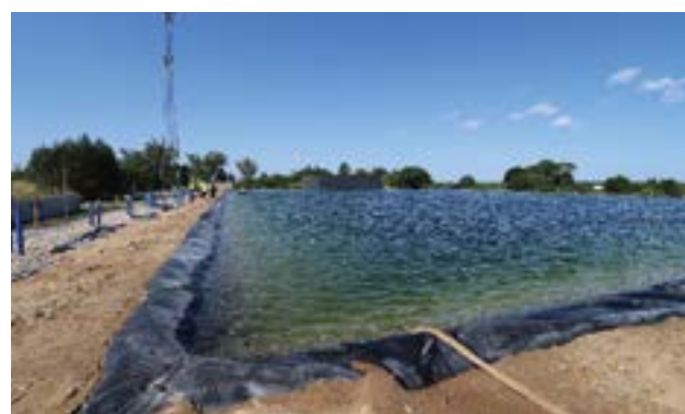
■ Seasonal heat storage filled with water before closing the top cover
