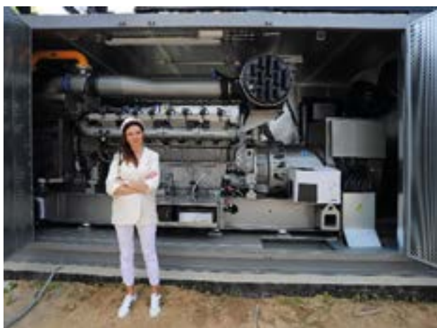
■ Cogeneration engine powered by biogas and biomethane running at peak demand
