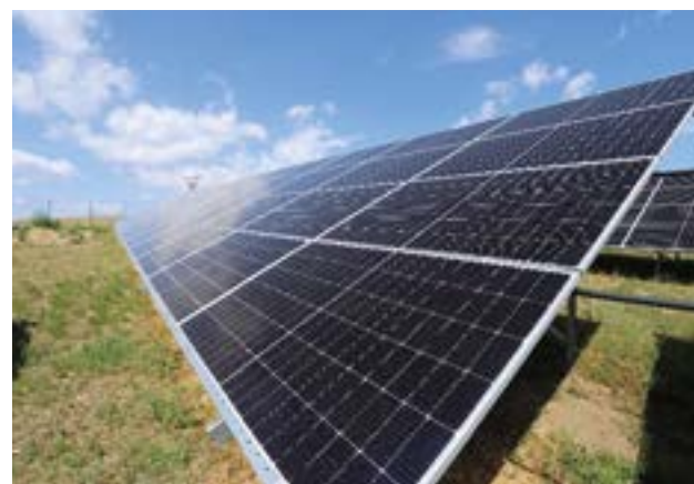
■ Photovoltaic farm powering a heating plant
