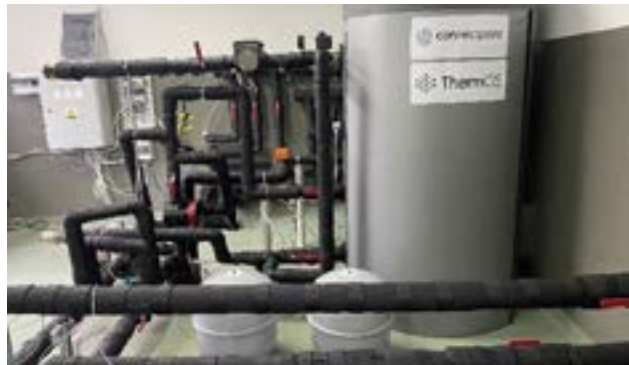
■ Equipped system buffer
