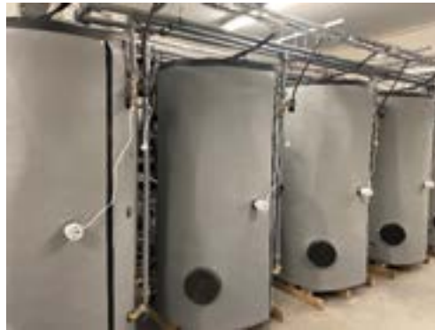
■ Phase-changing heat and cold storage facilities
