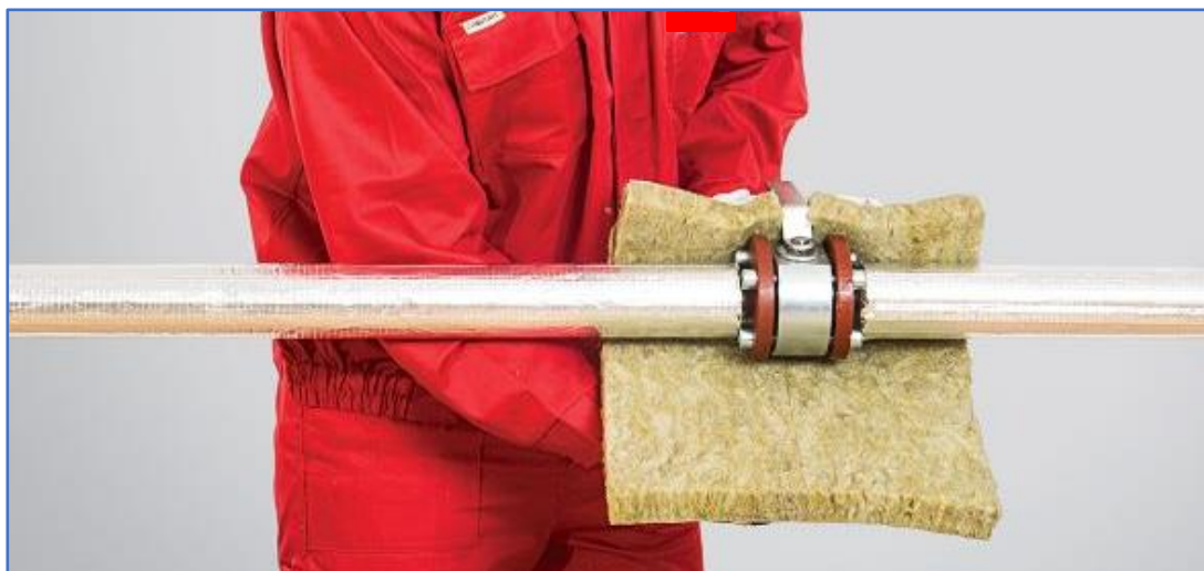
Pic. 2 centre of the insulation: securing the valve with a layer of insulation
