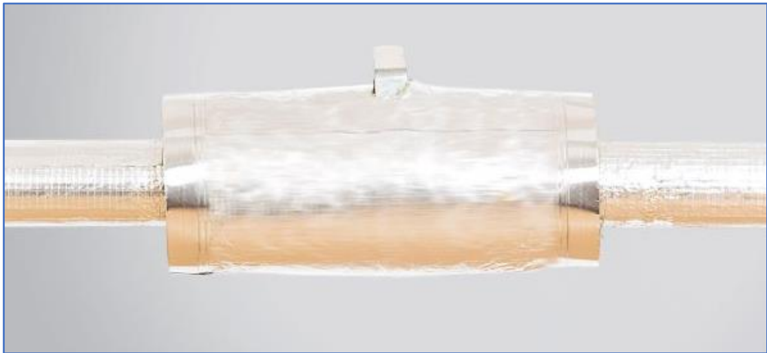
Pic. 4 centre of the insulation: a properly insulated valve
