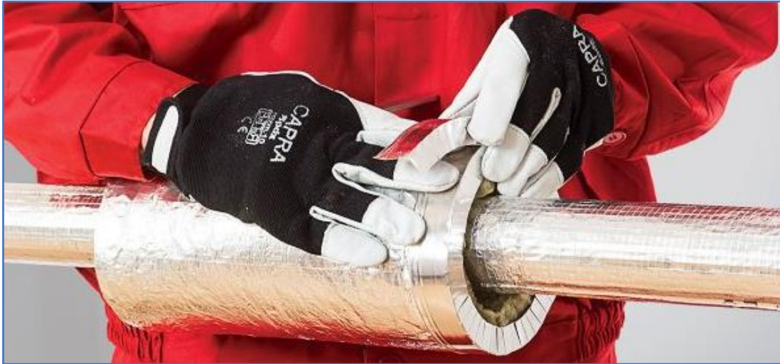
Pic. 3 centre of the insulation: securing the edges with a aluminium cuff
