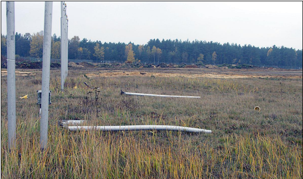
19 – Damage to the approach lights system ahead of EPKT RWY27 threshold after the accident
