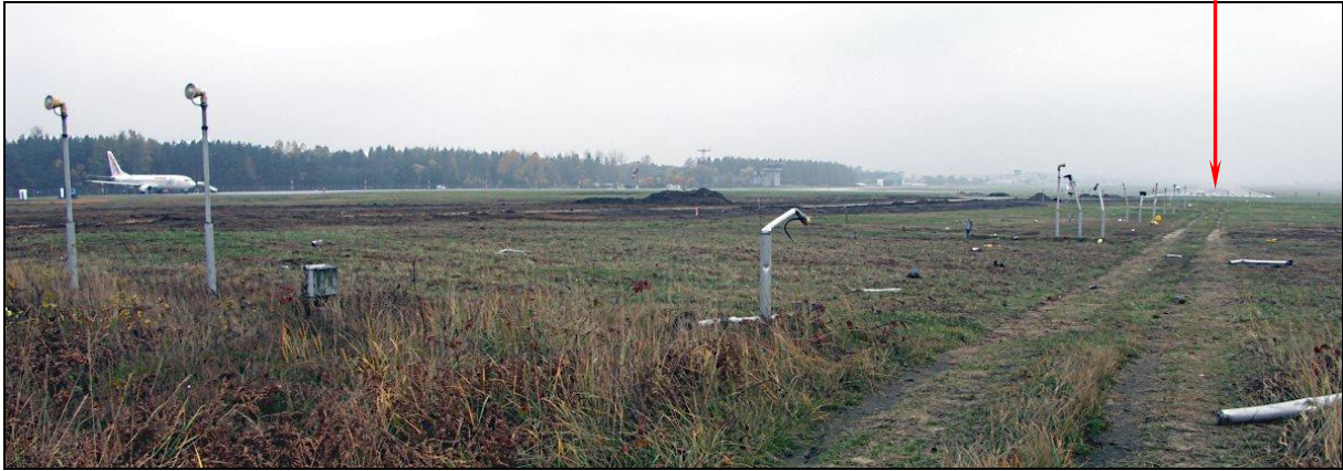
22 – Damage to the approach lights system ahead of EPKT RWY27 threshold after the accident. Visible RWY27 threshold
