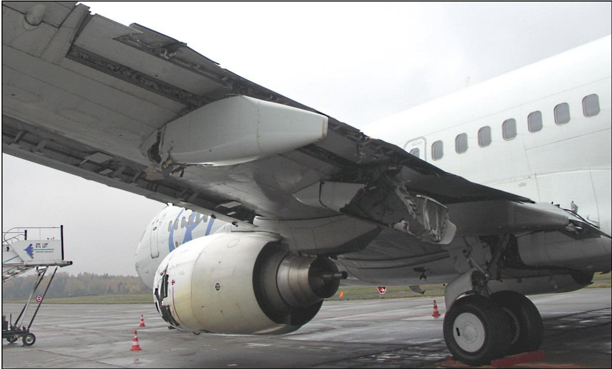
61 – Damage to the rear section of the left outboard flap and the flap track fairing – close-up
