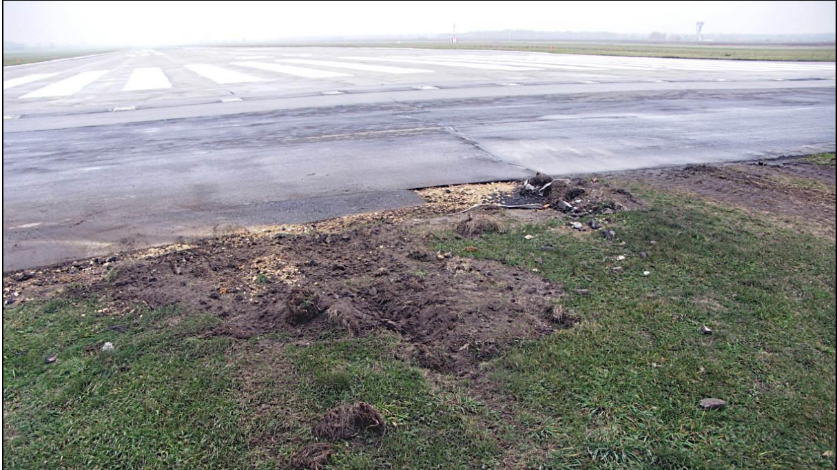
27 – Crossing point of the RWY27 threshold by the airplane left main landing gear wheels
