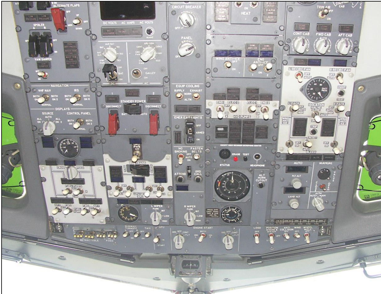
32 – Forward overhead cockpit panel
