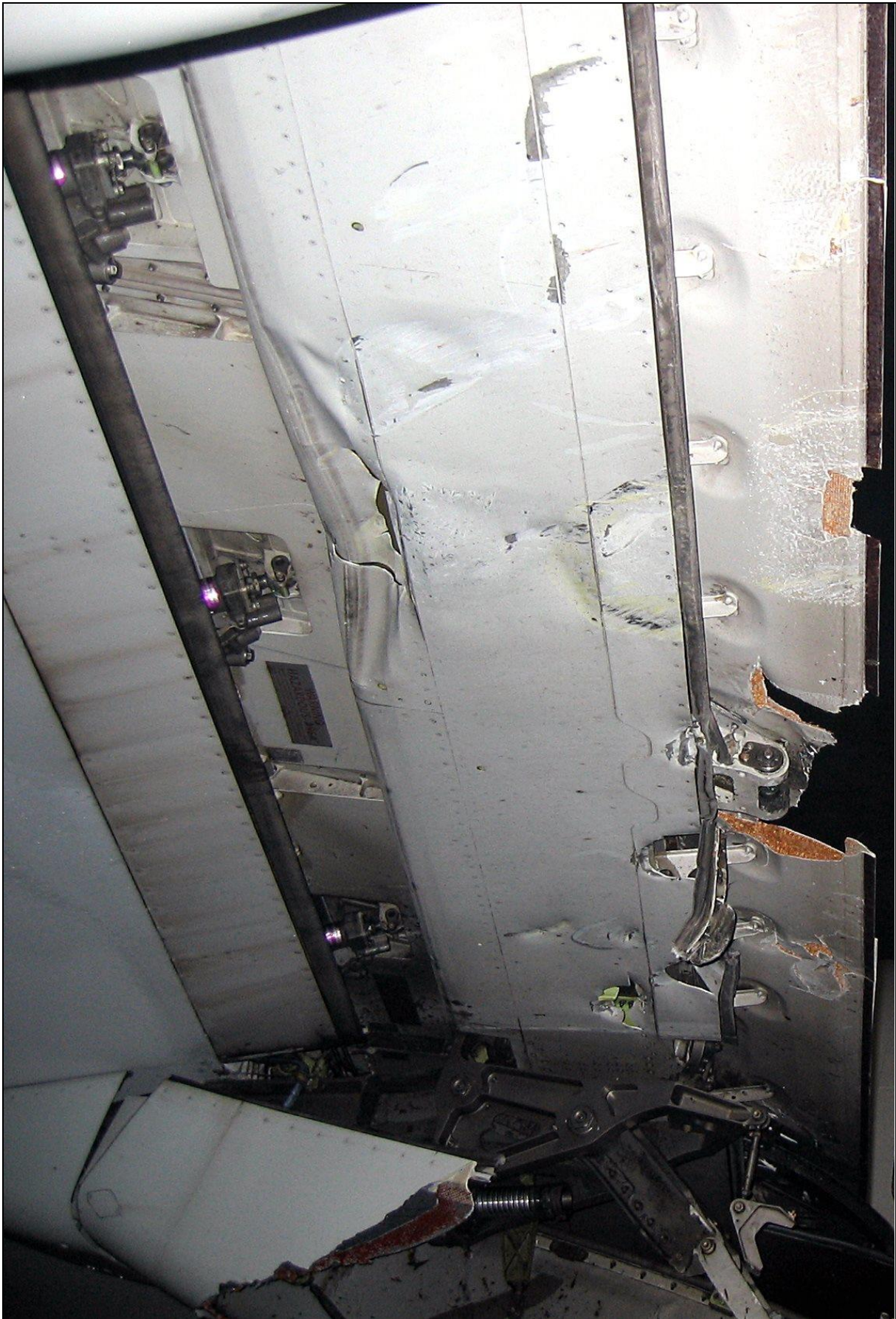
57 – Damage to the bottom of the left outboard flap – close-up [photo: airplane crew]
