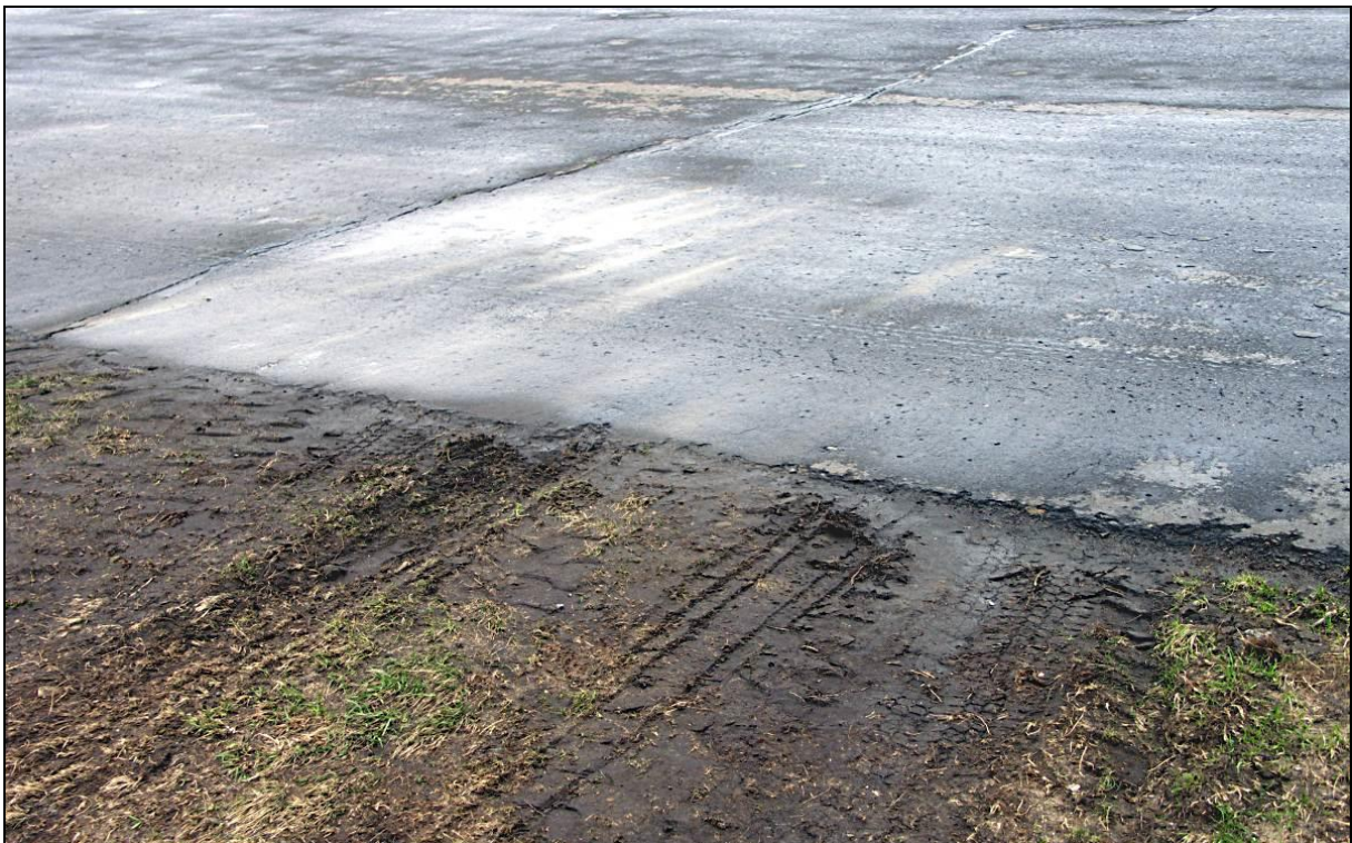
28 – Crossing point of the RWY27 threshold by the airplane right main landing gear wheels
