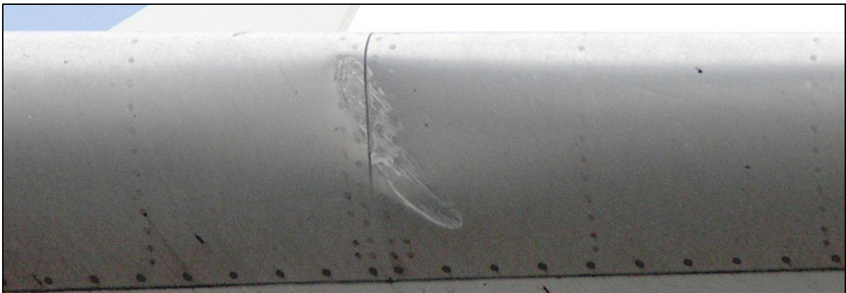
92 – Damage to the left horizontal stabilizer leading edge – close-up
