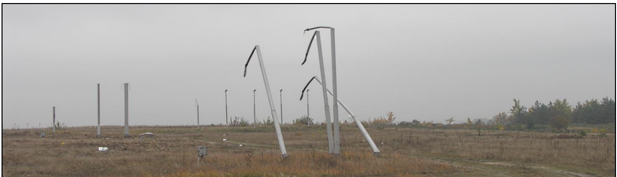
10 – Damage to the approach lights system ahead of EPKT RWY27 threshold after the accident
