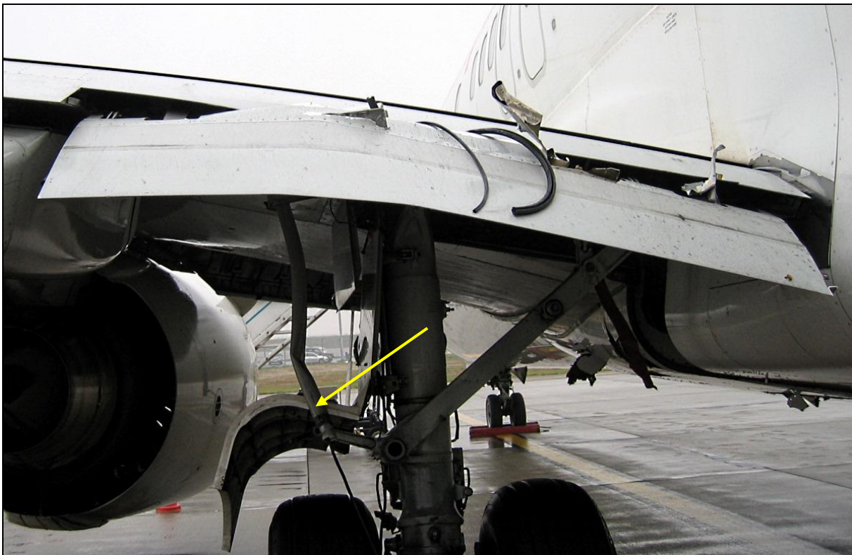
60 – Damage to the rear section of the left inboard flap – close-up. Arrows show the lights pieces stuck in the airplane structure [photo: airplane crew]
