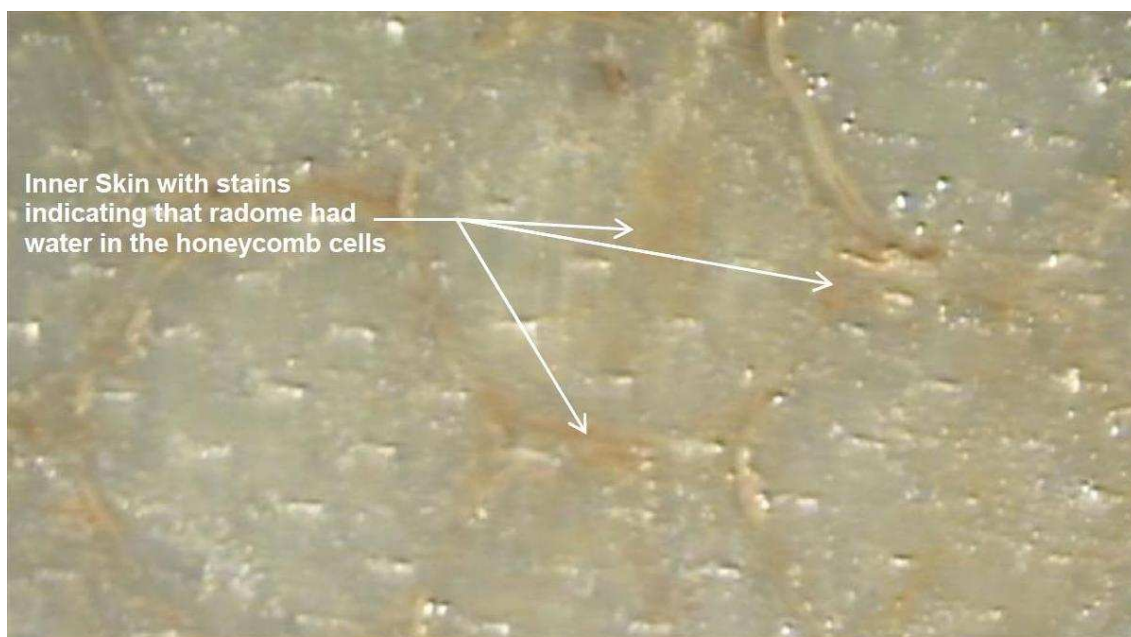
Figure 9 Contact Air Sample # 1, View Looking In Nose Section (Failure Area) Pattern Left by Honeycomb Material
