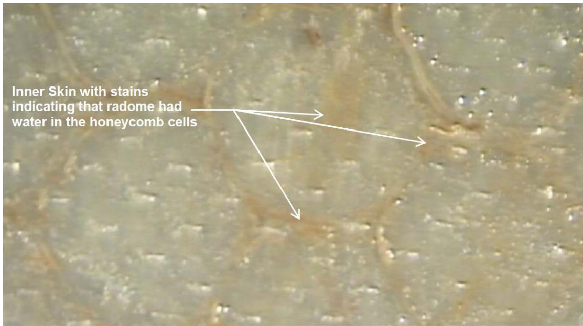
Figure 9 Contact Air Sample # 1, View Looking In Nose Section (Failure Area) Pattern Left by Honeycomb Material
